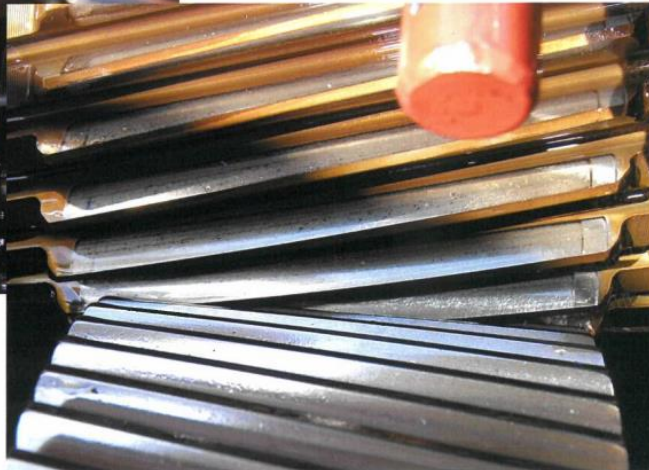
HS IMS pinion Marks from two running positions
